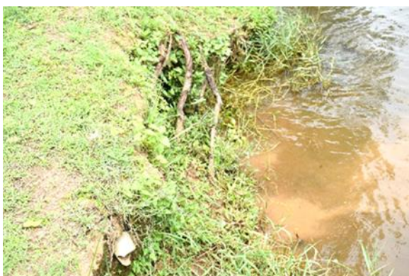
Eroded banks in Kotte Canal
